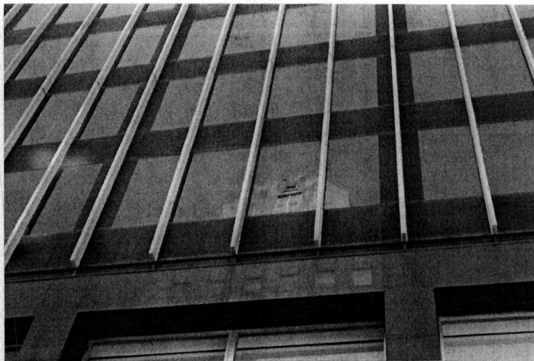
Fig. 7 (above). Detail of front elevation showing black granite base and upper wall surface with mullions
