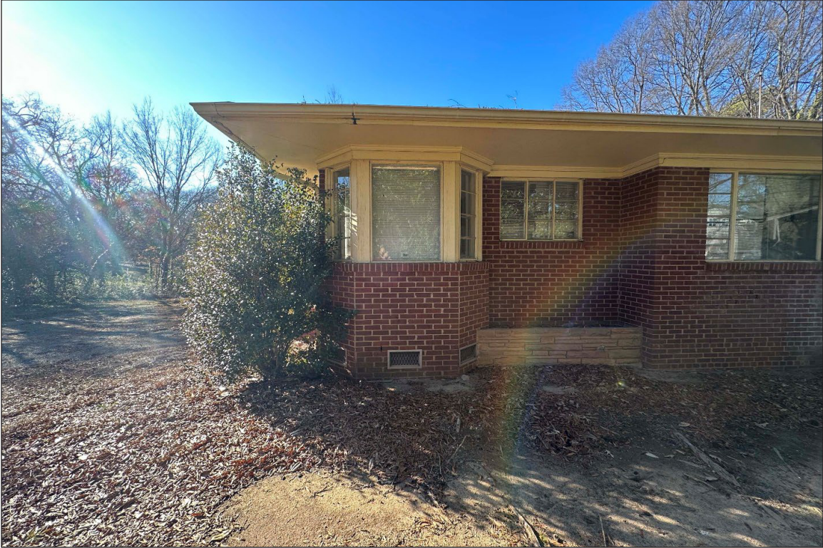
Photo 05: 1011 Oberlin Rd, Raleigh, NC (01/10/2023) Perspective of east entry showing by window in the background, facing west.
