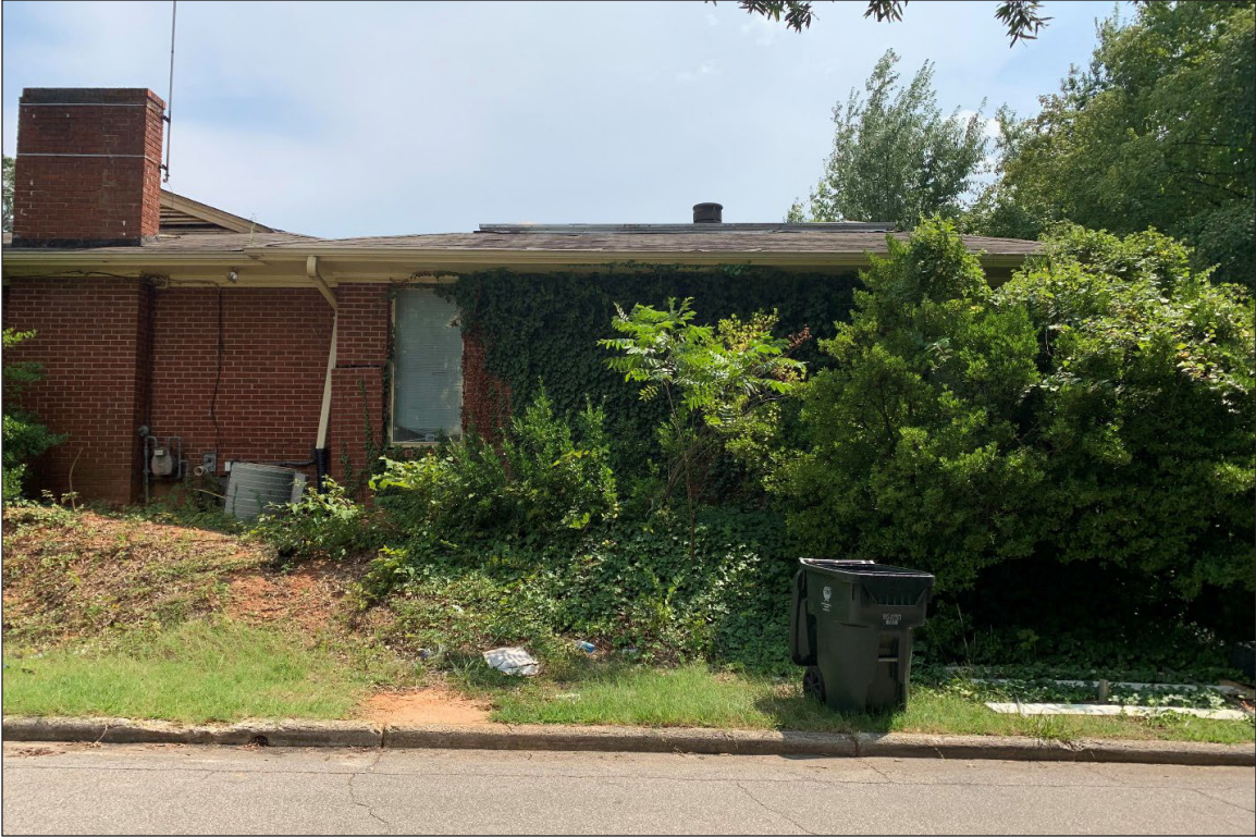
Photo 17: 1011 Oberlin Rd, Raleigh, NC (08/10/2021) Perspective view of the north side of structure from Mayview Rd, facing south.
