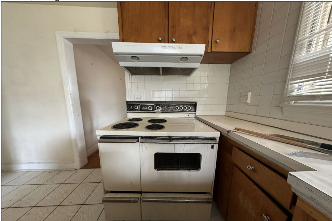
Photo 26: 1011 Oberlin Rd, Raleigh, NC (01/10/2023) Interior photo of the kitchen facing west showing original stove and cabinetry.
