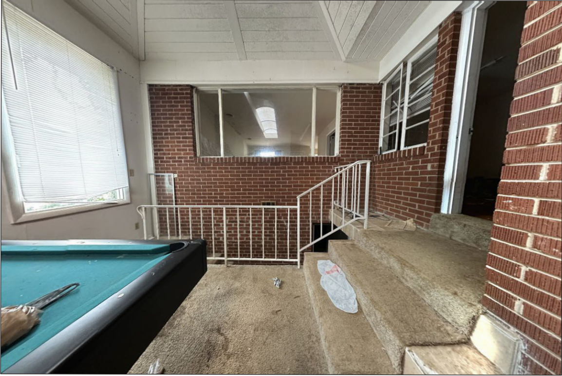
Photo 23: 1011 Oberlin Rd, Raleigh, NC (01/10/2023) Interior photo of the addition (former porch) facing east toward front living room.
