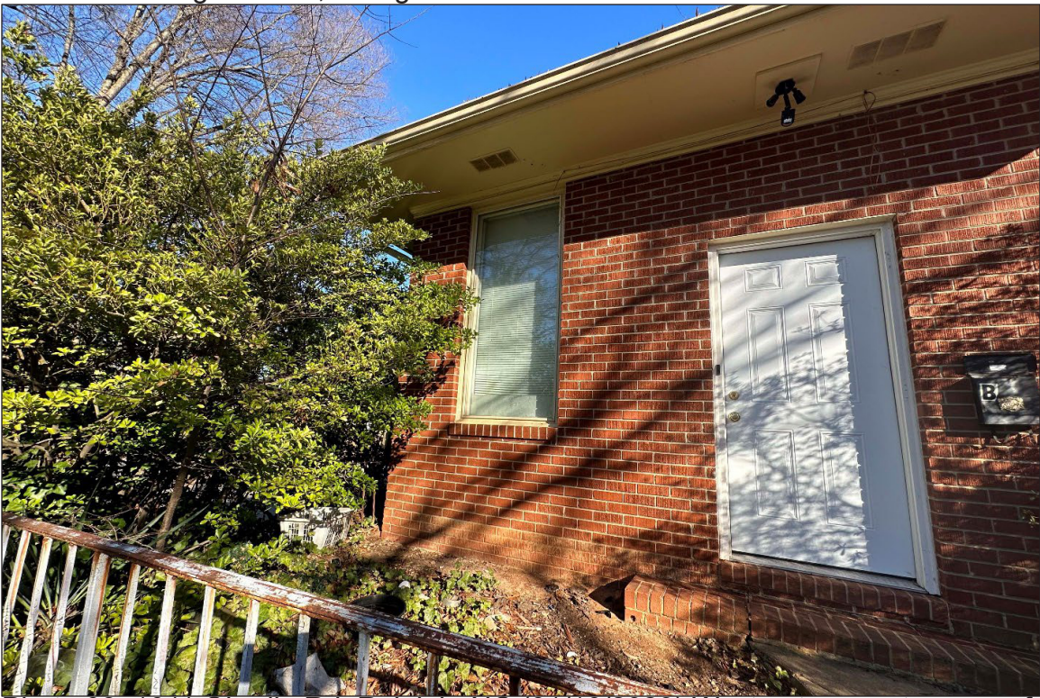
Photo 08: 1011 Oberlin Rd, Raleigh, NC (01/10/2023) West entrance at corner of addition, facing east.
