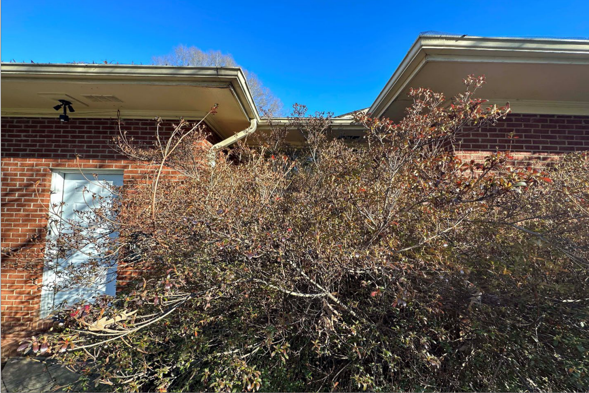
Photo 09: 1011 Oberlin Rd, Raleigh, NC (01/10/2023) West entrance with original structure beyond on the right of frame, facing east.
