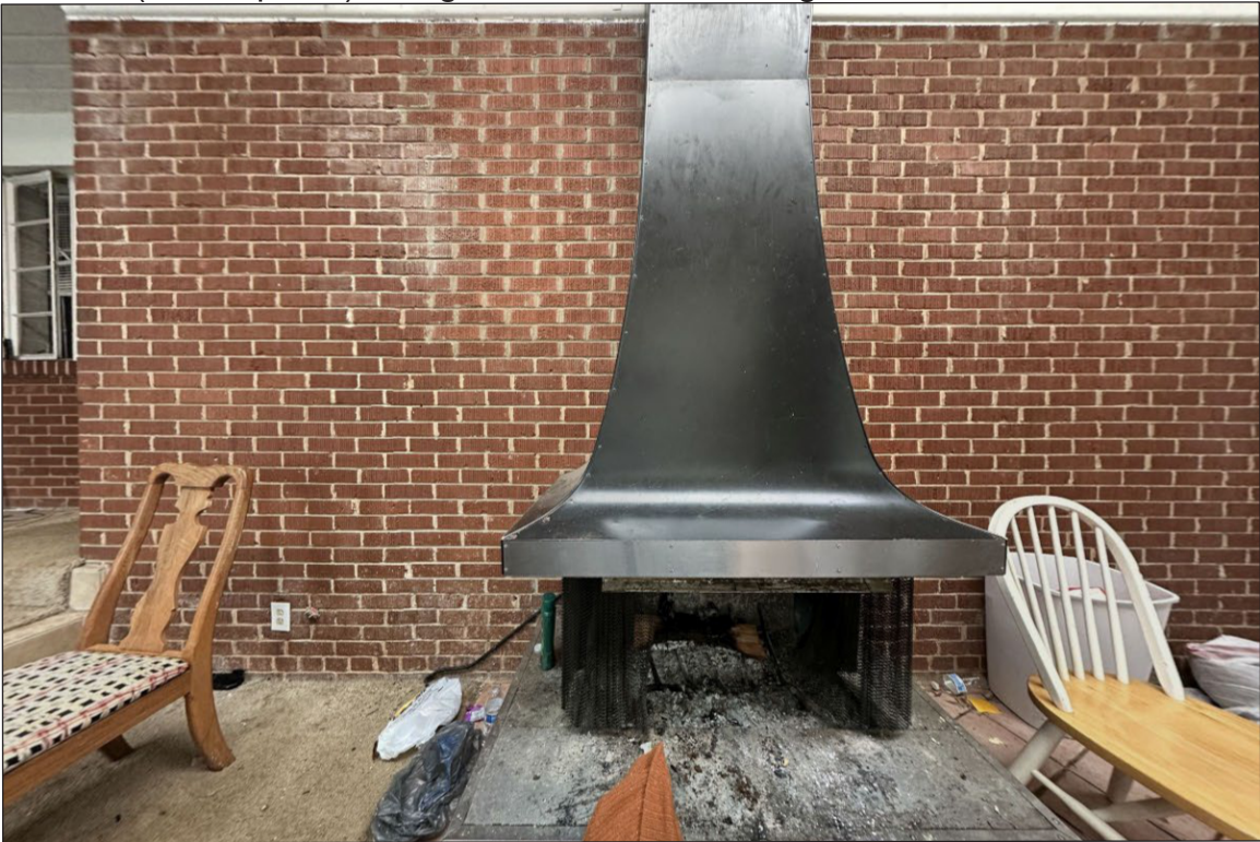
Photo 24: 1011 Oberlin Rd, Raleigh, NC (01/10/2023) Interior photo from within the addition facing south with the wood-burning fireplace at center.
