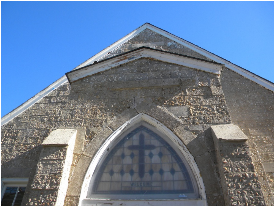
Figure 4. Detail of the gothic arched window, 1950s or 1960s stained glass, and buttresses.
