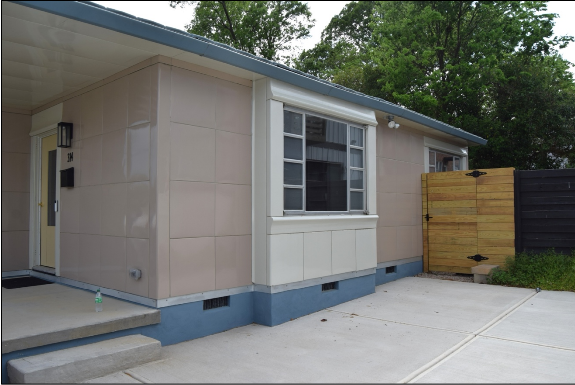
Photo 4. N side elevation showing living room bay window at center, view SW.
