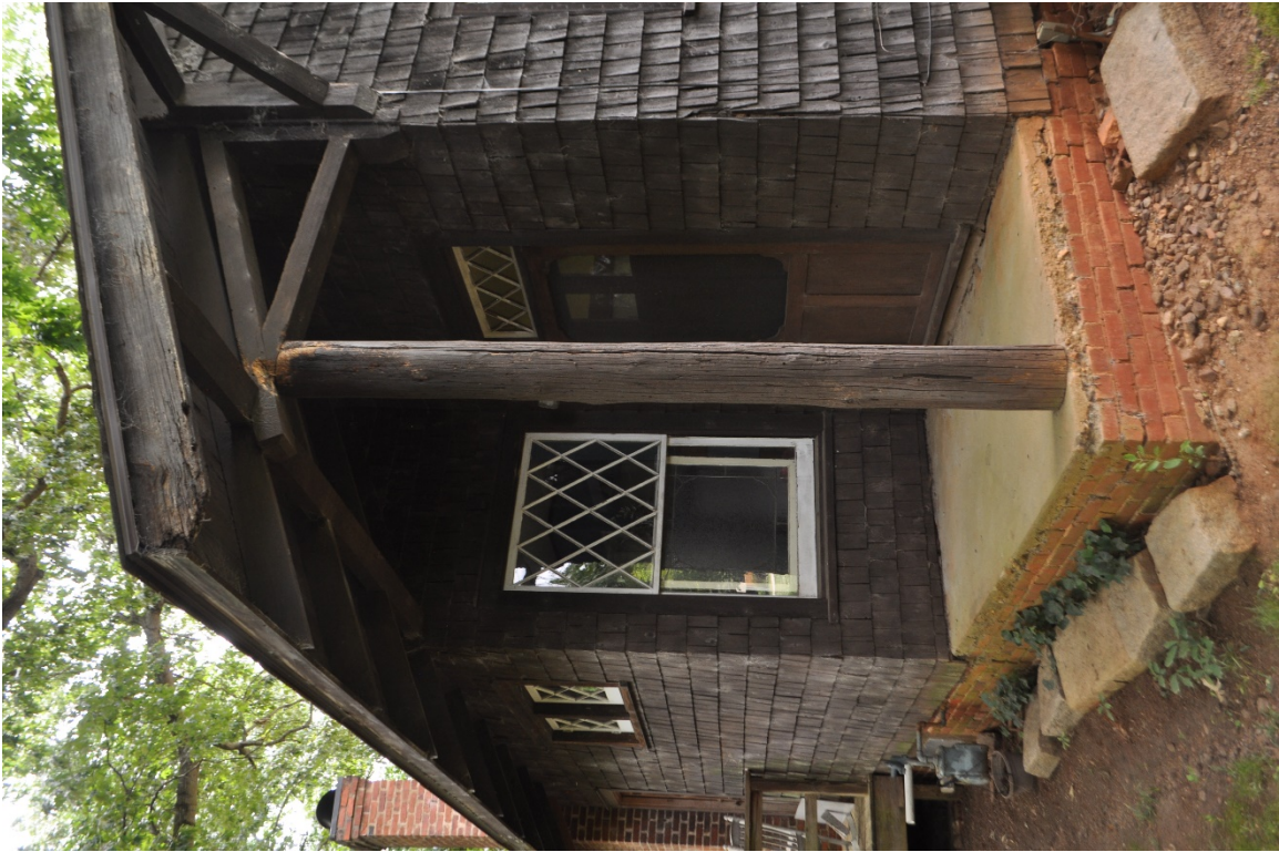
Plate 11: Detail view of the inset porch on the northwest corner of the house.
