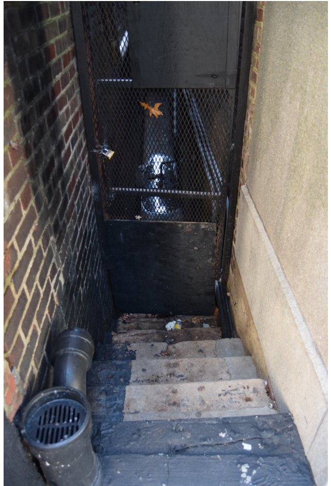
Sir Walter Raleigh Hotel, 400 Fayetteville St., Alley between Sir Walter Raleigh Hotel (at right) and neighboring building, view W. looking down the stairs.
