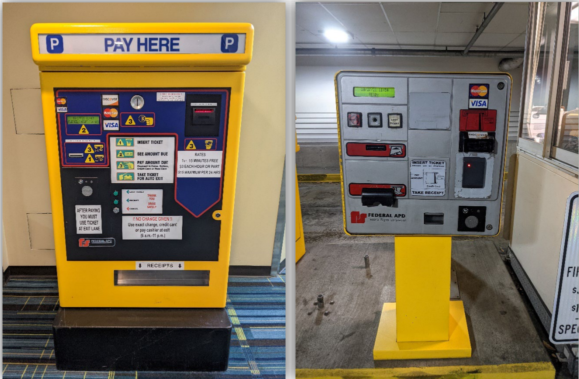
(Current pay on foot station and lane equipment in Convention Center Parking Deck)
