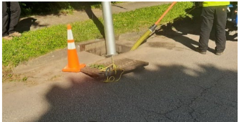
Photo 5. Elevated catch basin causing pooling of water on Jacqueline Lane.
