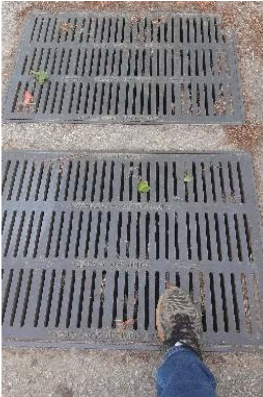
Photo 3. Existing storm drainage grates with poor grate spacing on the north side of Jacqueline Lane.
