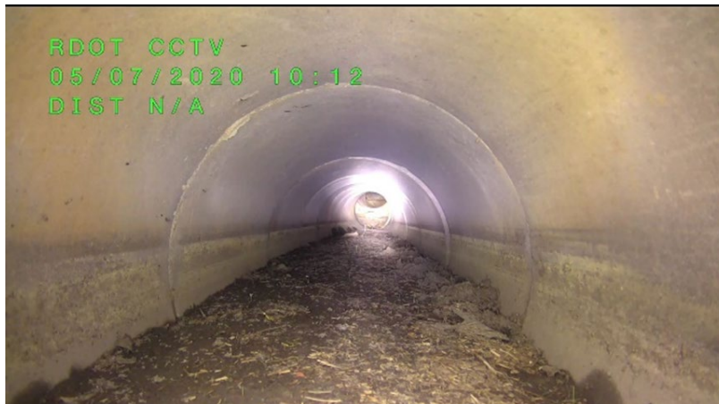
Photo 1. Sediment buildup in the stormwater pipes under Jacqueline Lane.
