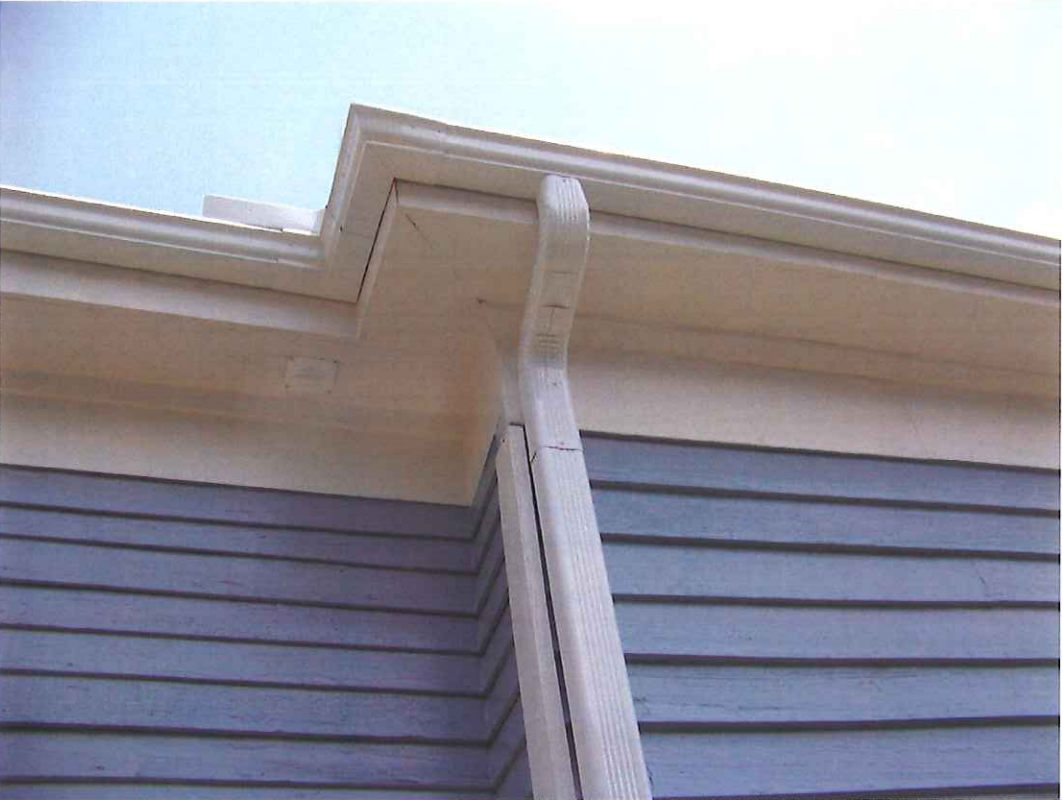
Trim transition from crown molding to flat band at existing addition to original structure
