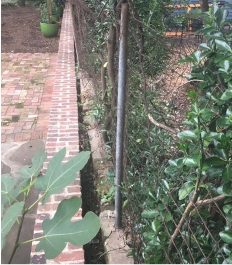
This is the back lot line and shows where the new fence will sit behind the retaining wall.
