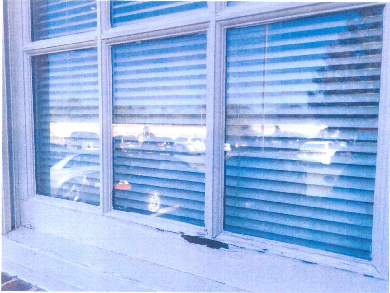
Exhibit 3: Example of rotten wood in window at Pilot Mill. The far light on the left has failed too.
