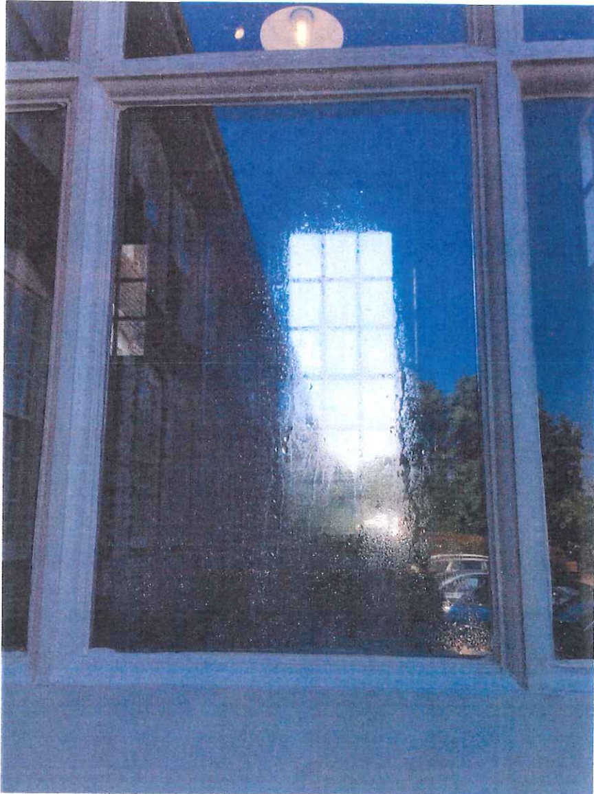
Exhibit 2: Example of failed insulated glass. Leak in the seal causes condensation between the two pieces of glass.
