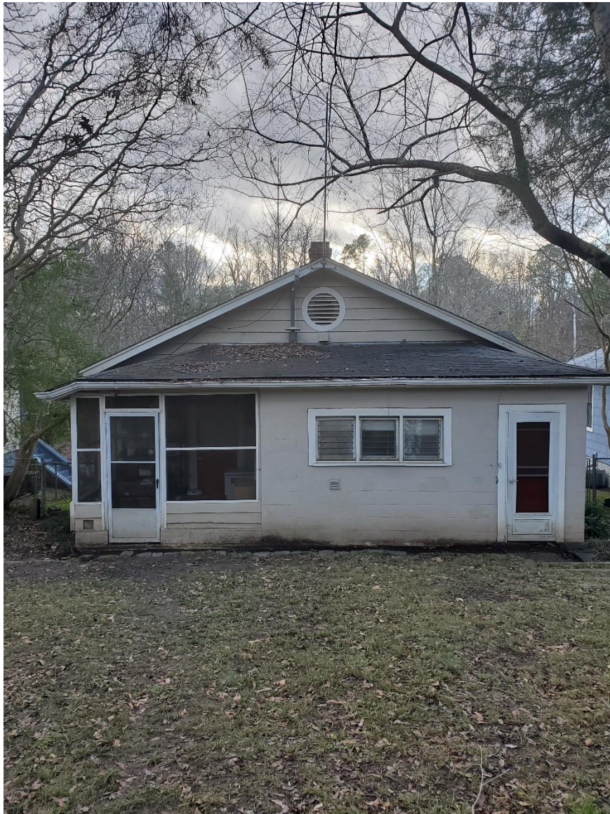
Photograph #2: Rear of House – CMU/ Screen Porch to be Removed (East Elevation)
