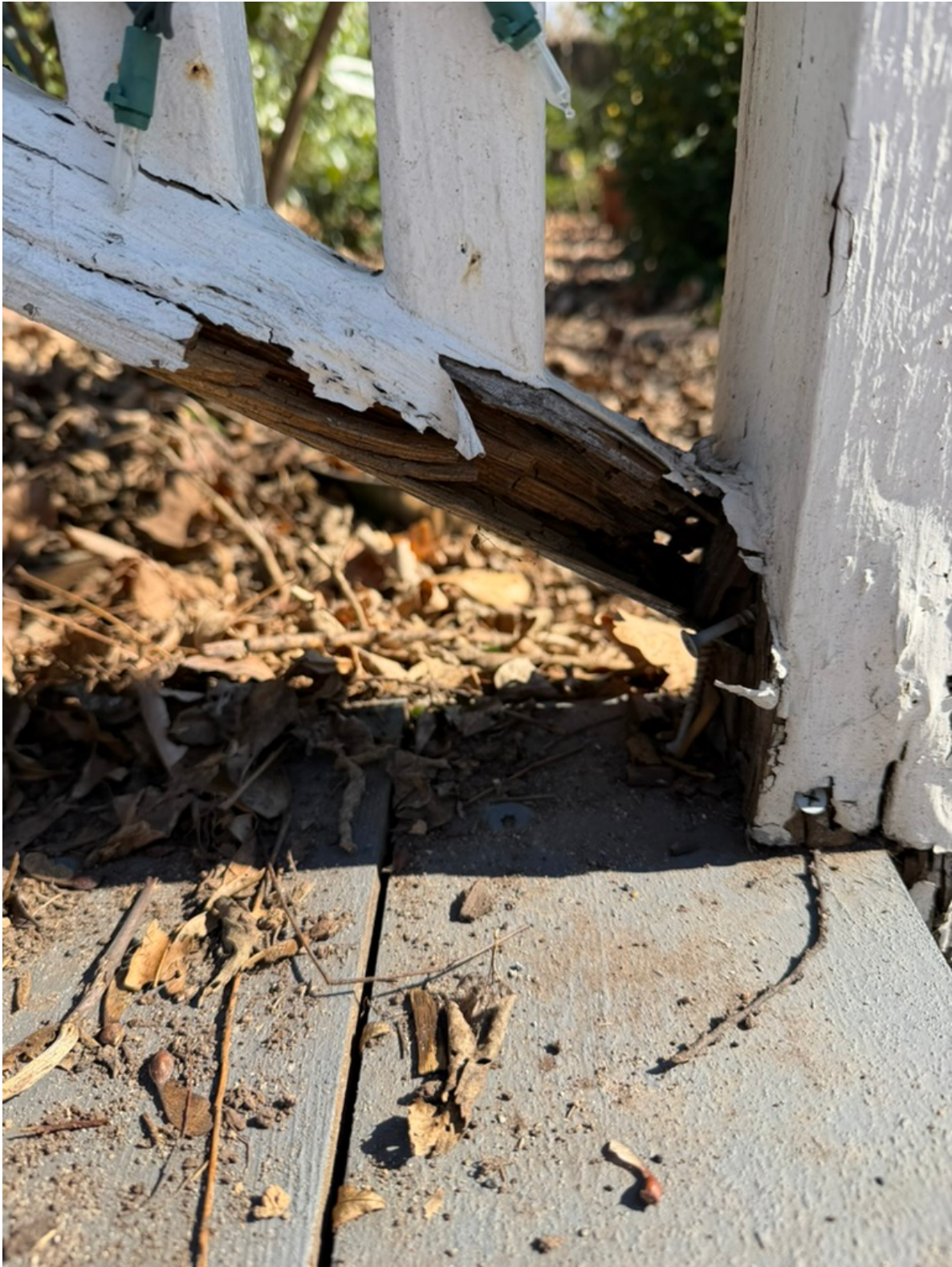
Rotting railings (528 E Jones)
