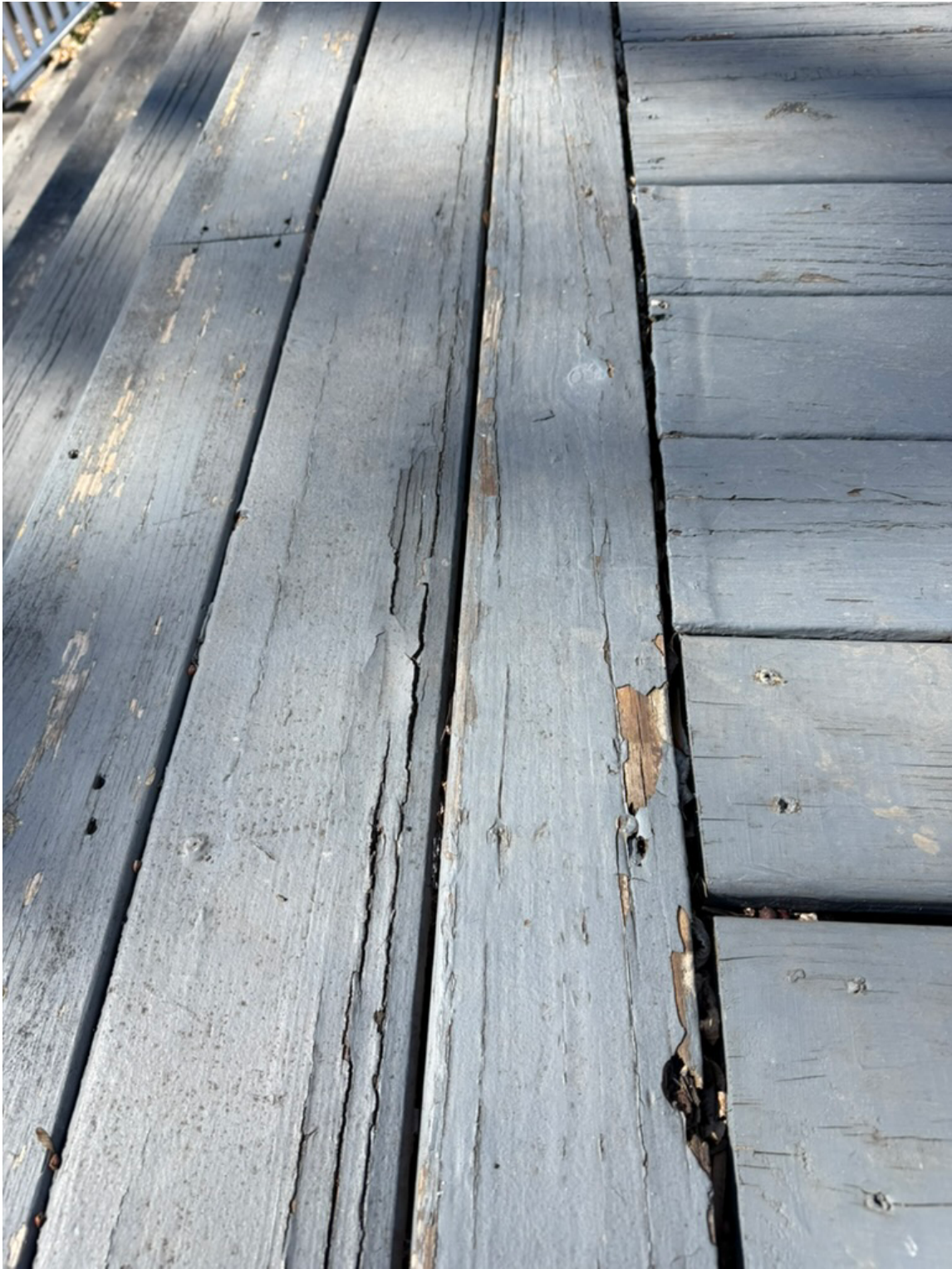
Peeling, damaged deck boards (528 E Jones)
