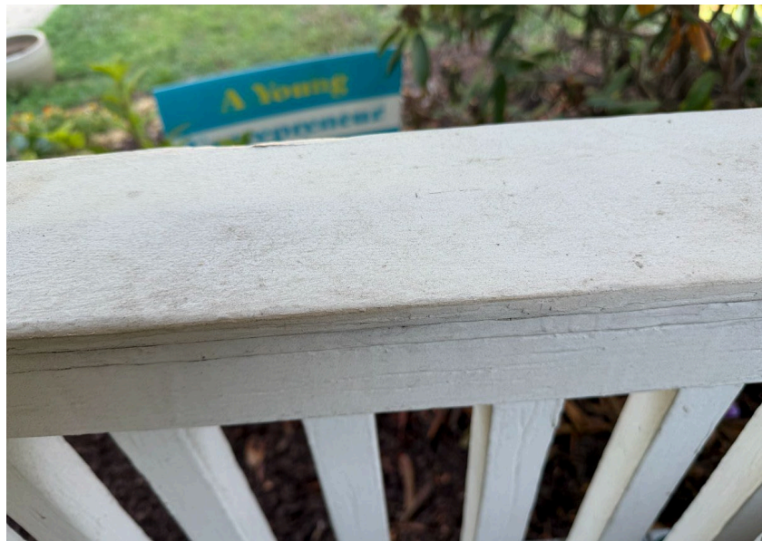
Existing front porch cap profile — note the eased edge and overhang reveal to be replicated.
