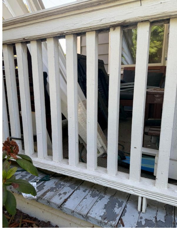
Existing front porch railing — overall view of cap, square slat balusters, and bottom rail.
