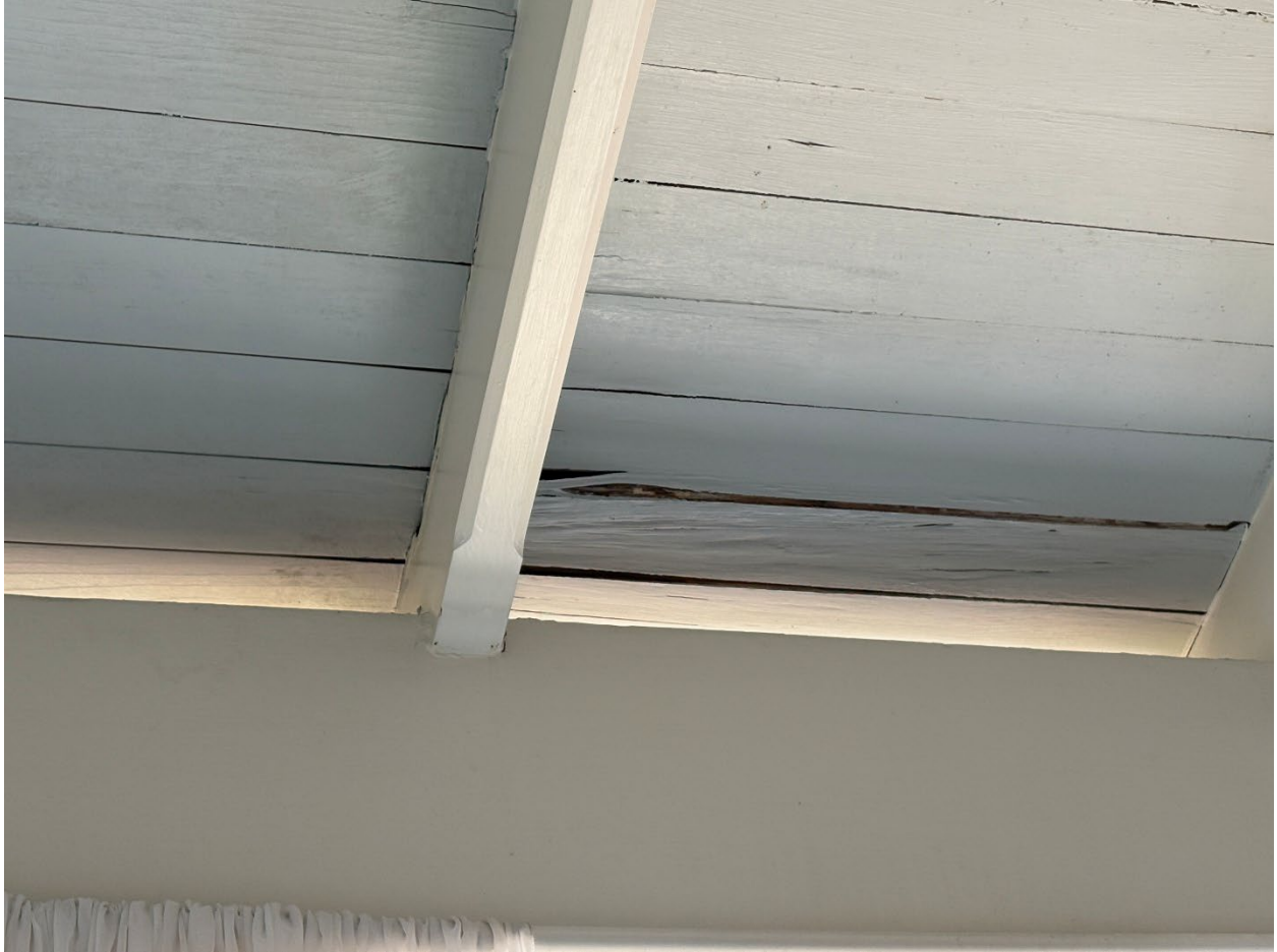
Figure 2: Rotting tung and groove porch ceiling at 514 Oakwood Ave.
