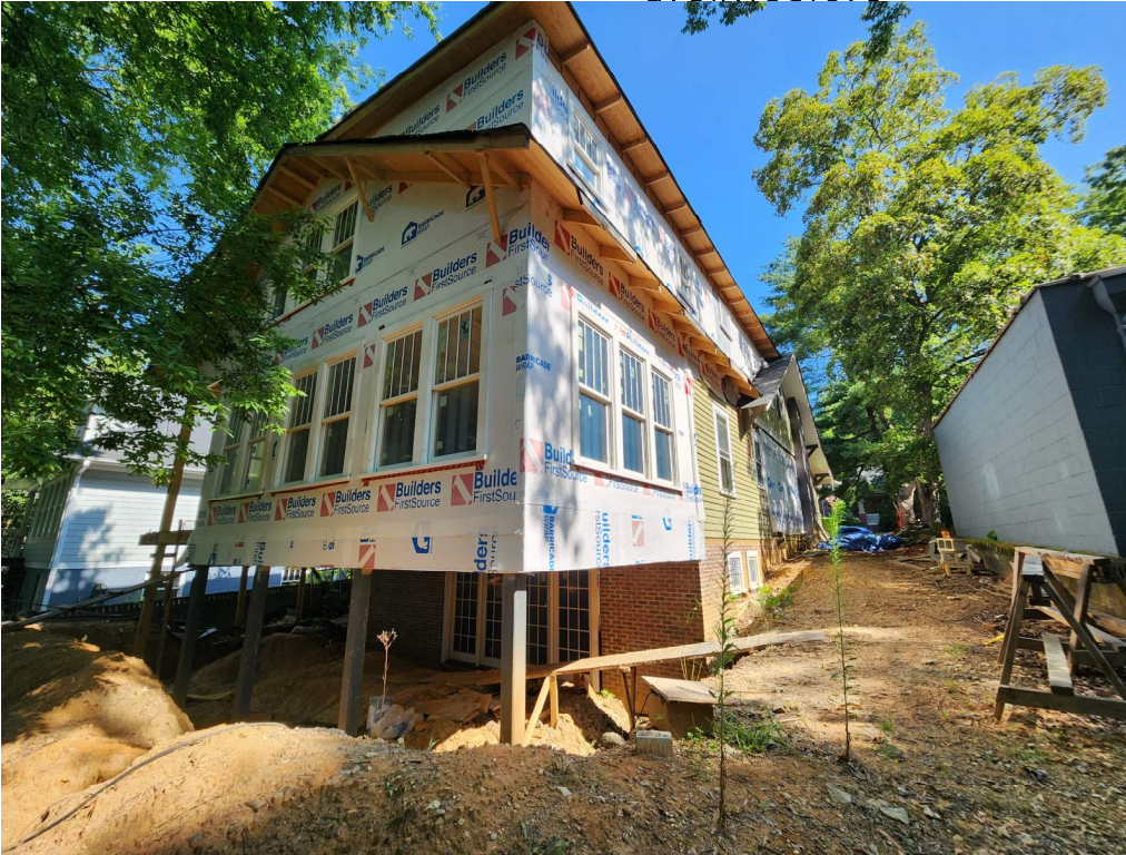
9-Southeast view of addition showing grade and need for 5'h retaining wall.
