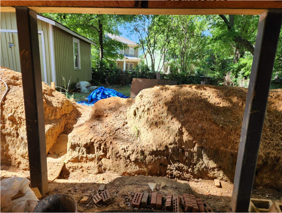
7-South view of Covered Patio before final grading showing location of proposed stairs to grade.
