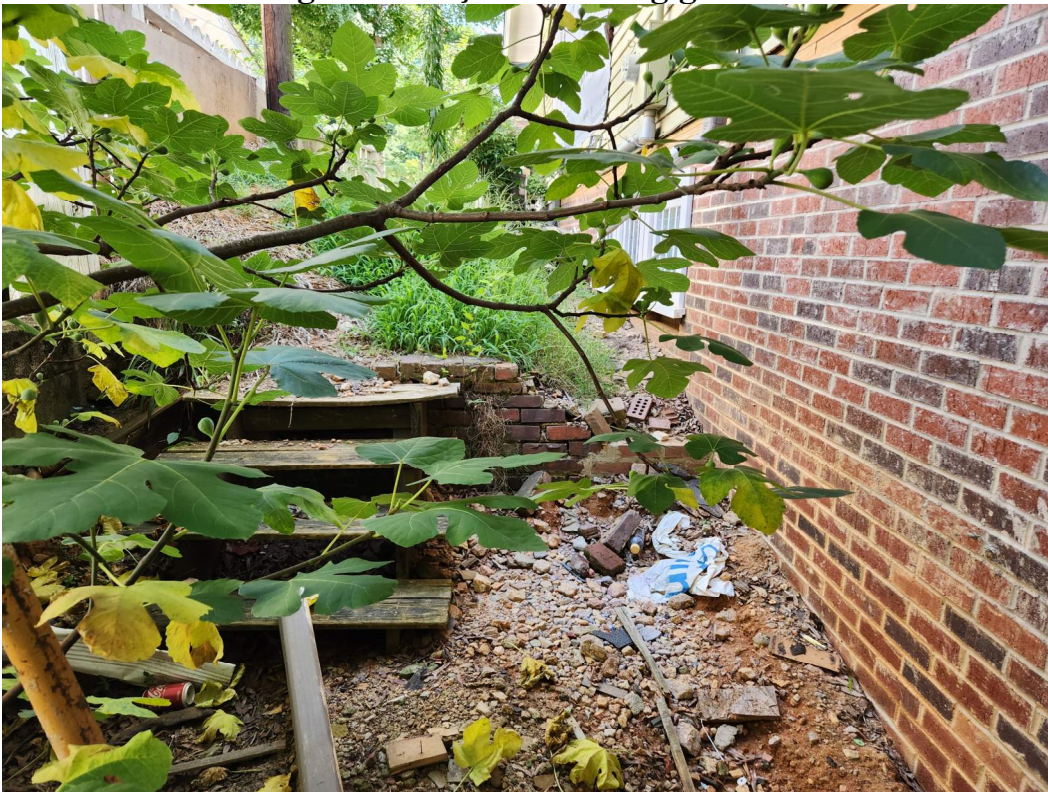
4-View deteriorated retaining wall and existing landscape stair to be removed.
