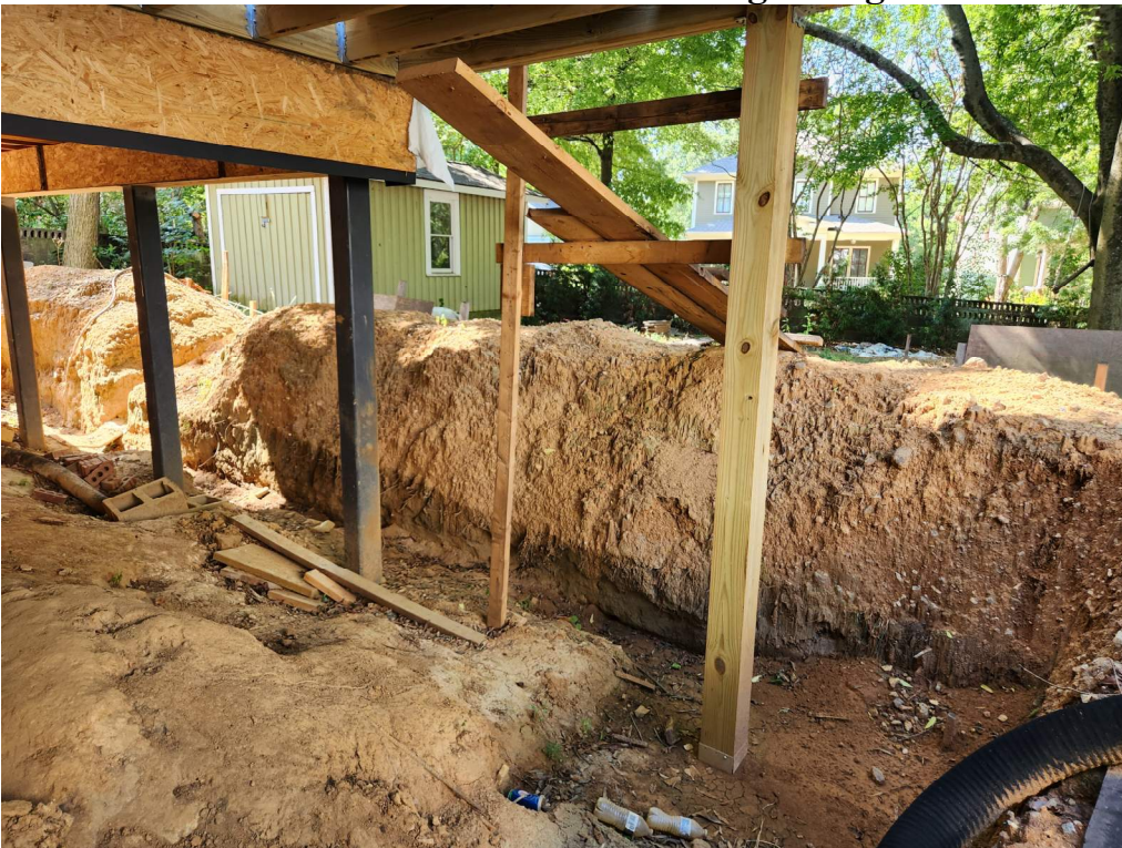
6-South view of Covered Patio before final grading to backyard showing need for 2' retaining wall
