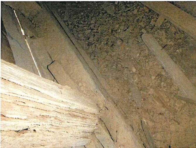
Interior of attic showing damage
