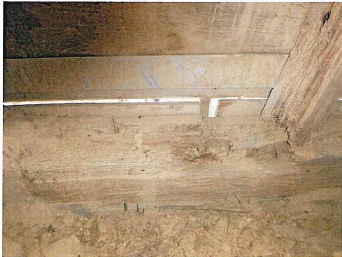
Interior of attic showing damage
