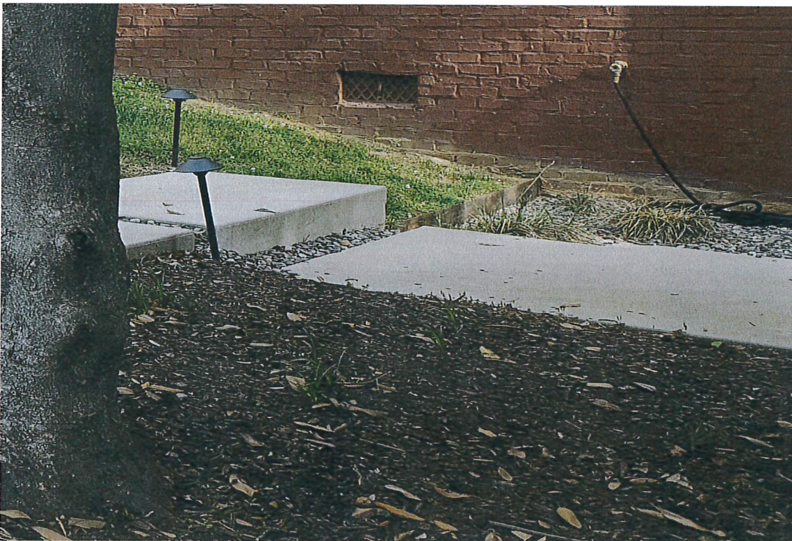
Photo of Existing Broom Finish Concrete Steps Proposed steps to match existing.
