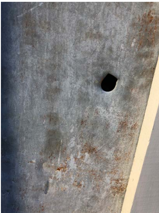
Many bullet holes through metal siding of shed
