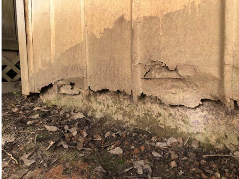
Deteriorating metal siding
