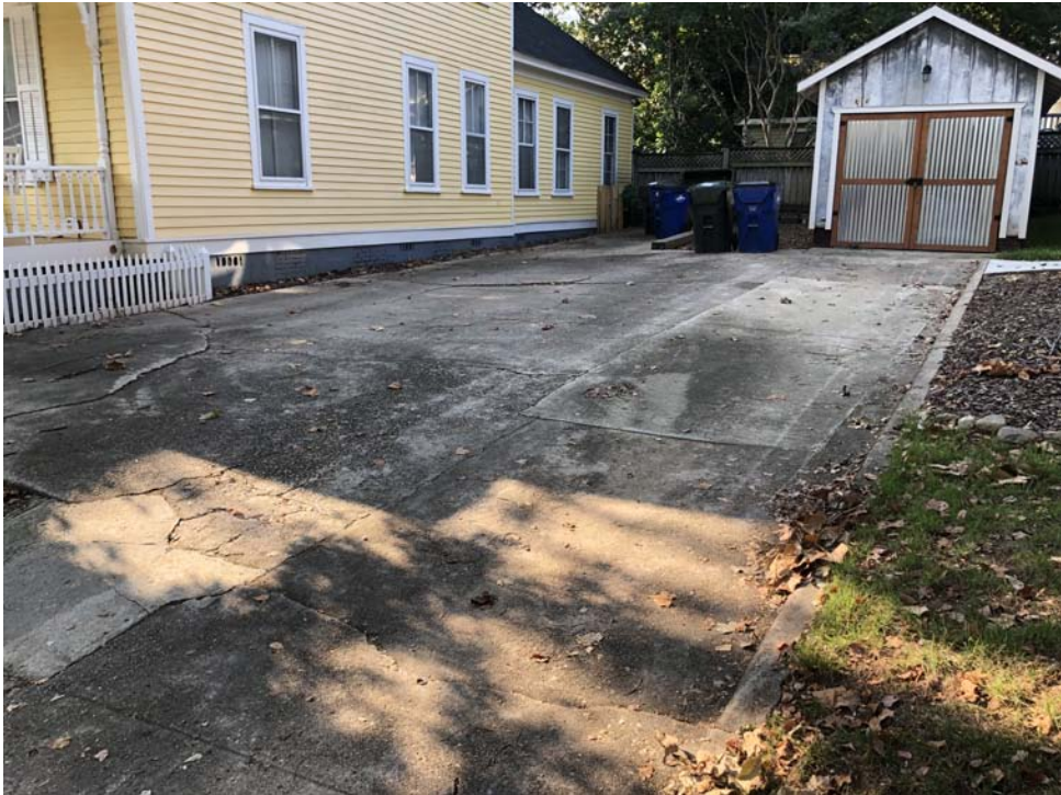
Existing concrete pavement, large and deteriorated
