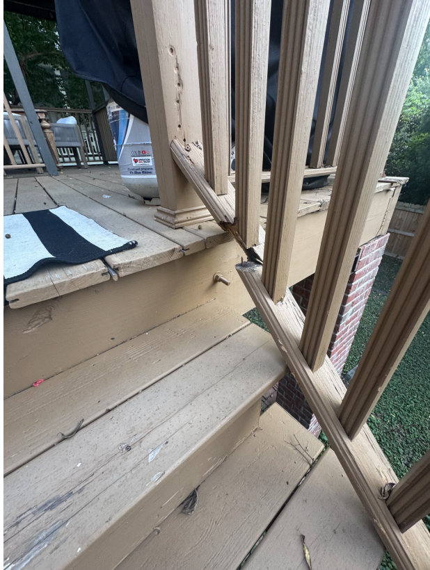
Evidence of rotting wood on the stairs.
