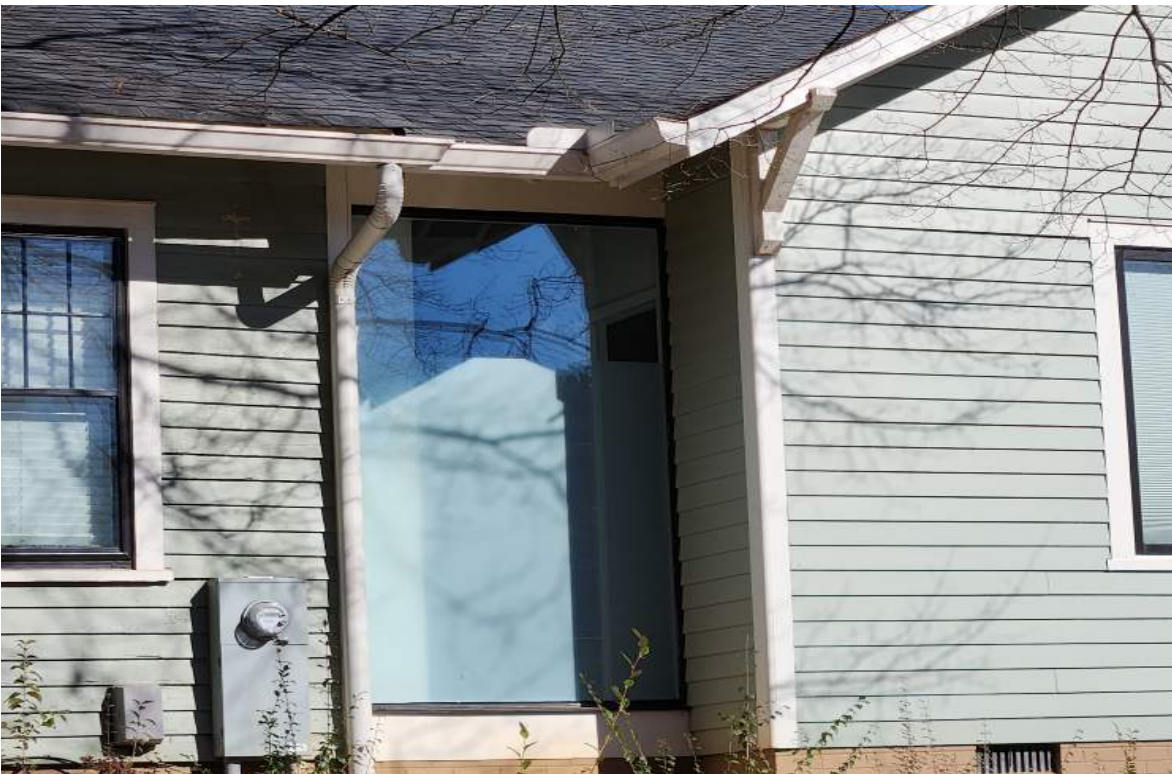
02- 1100 Filmore Street- Detailed view of glassed-in connector. This “glass” wall uses glass as the connecting material. While glass is found everywhere in the district, this new use of a historic material not based on any precedents in neighborhood was approved with COA application # 189-16-CA.
