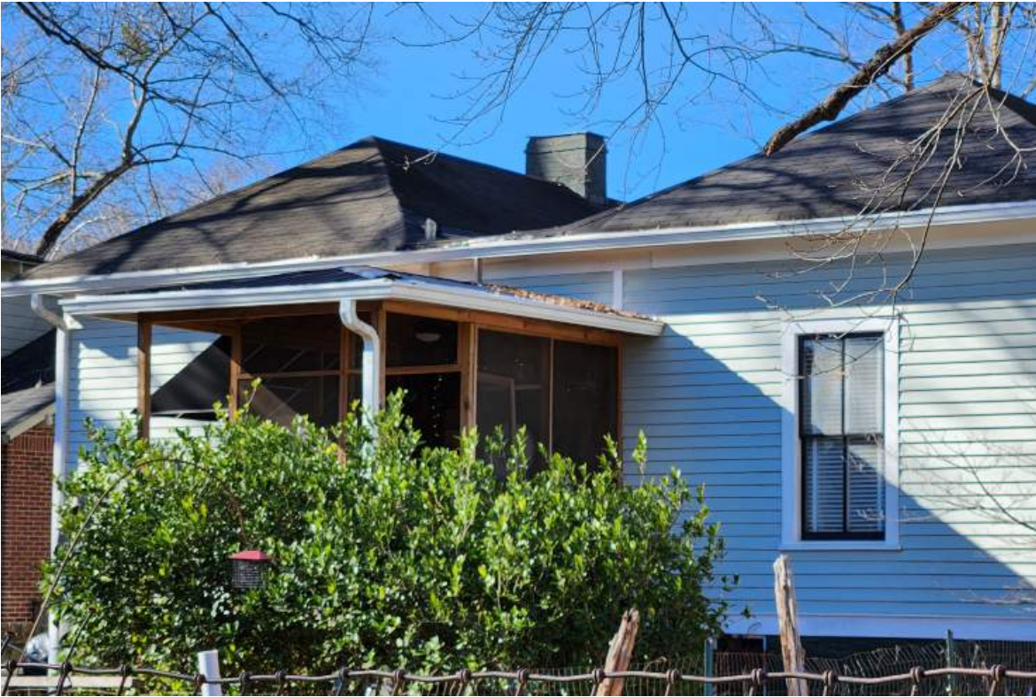
05- 1214 Glenwood Ave- Low slope roof addition dropped below existing eave.
