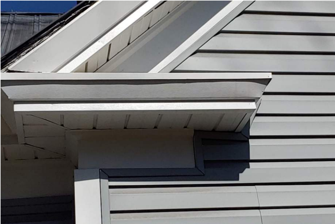
09- View of existing eave detail showing layers of roofing beneath metal roof
