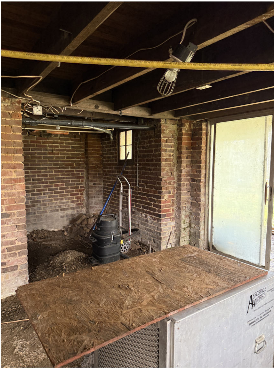
View of the existing windows and sliding doors from inside the crawlspace
