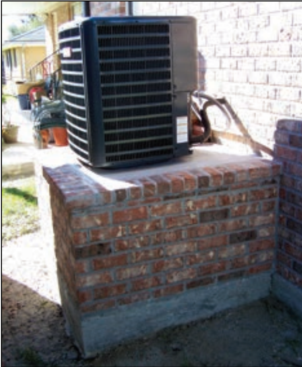
Figure 3-1. Air conditioning compressor elevated on a pedestal.
