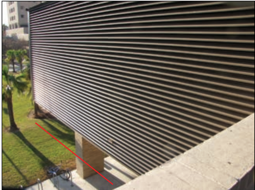
Figure 5-14. Example of protected emergency power system components. The BFE (shown approximately in red) is below the second floor so primary components of the electrical system were elevated well above the required flood elevation.
