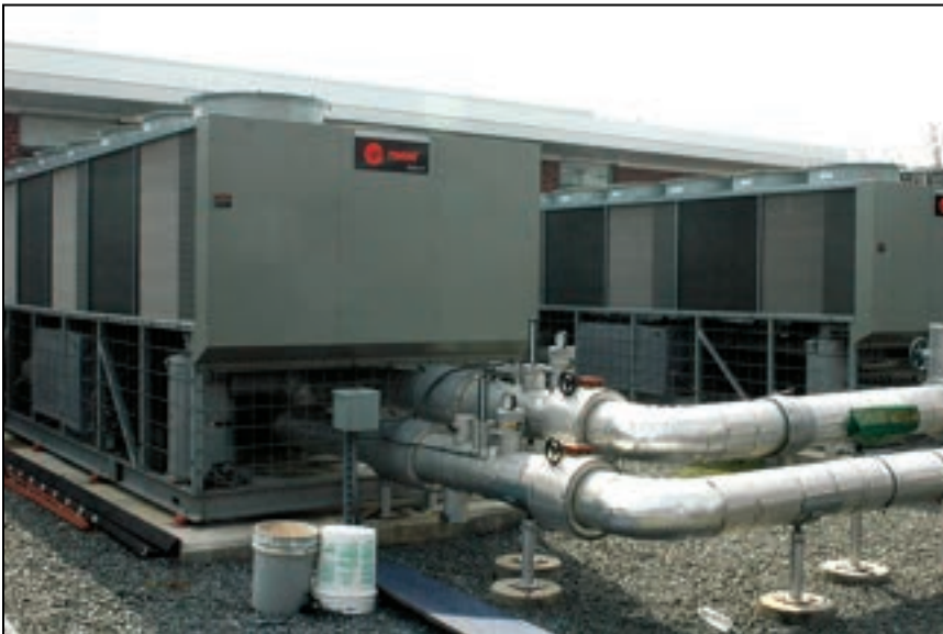
Figure 5-3. Air-Cooled rooftop chiller in Georgetown, Delaware.
