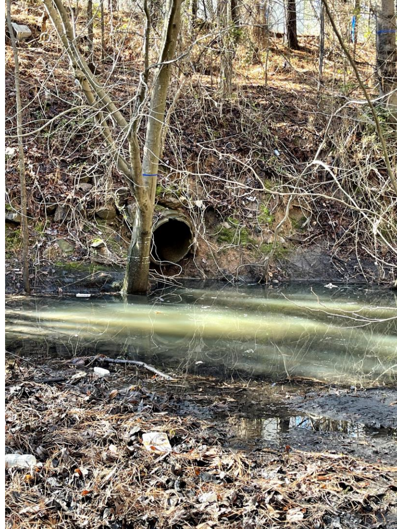
Figure 2: Impaired outlet structure function.
