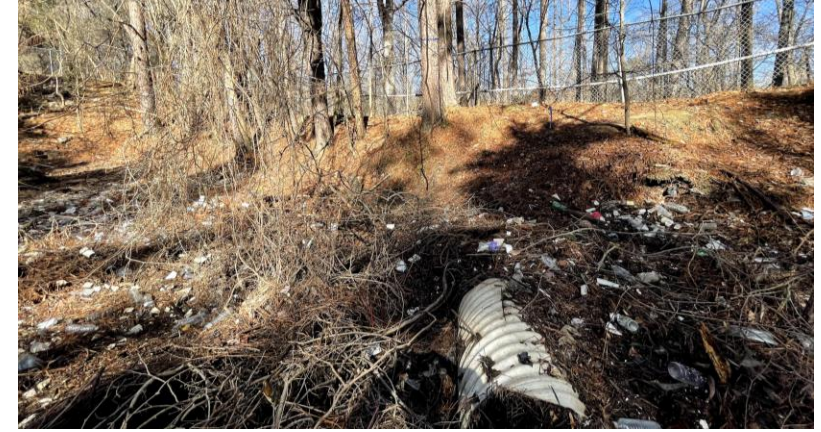
Figure 3: Erosion on interior and exterior slopes.
