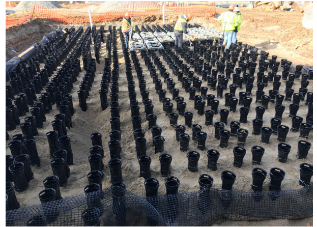
Silva Cell stormwater device located at John Chavis Memorial Park during construction.
