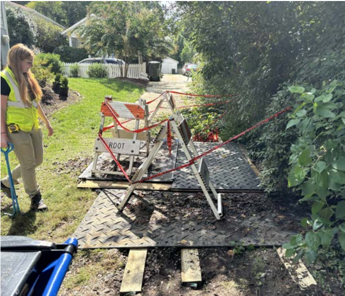
Sink Hole Covered on Creston Road
