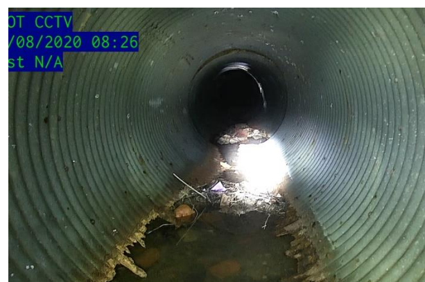
Rusted corrugated metal pipe bottom
