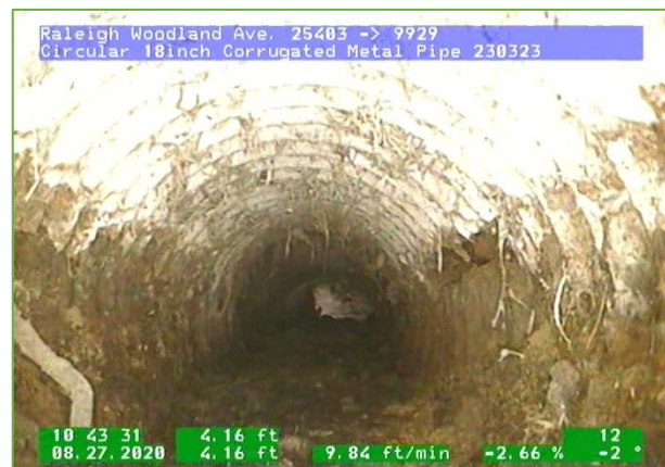
Sediment/deteriorated corrugated metal pipe
