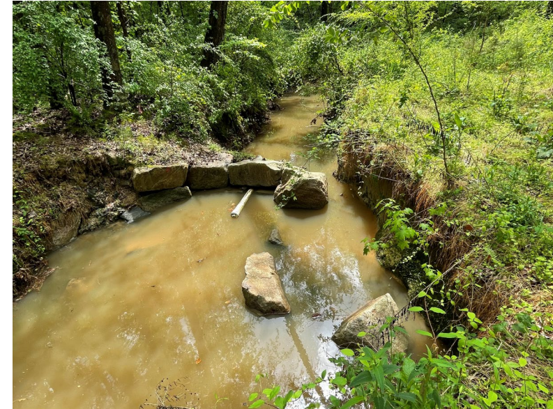
Damaged in-stream structure 2023
