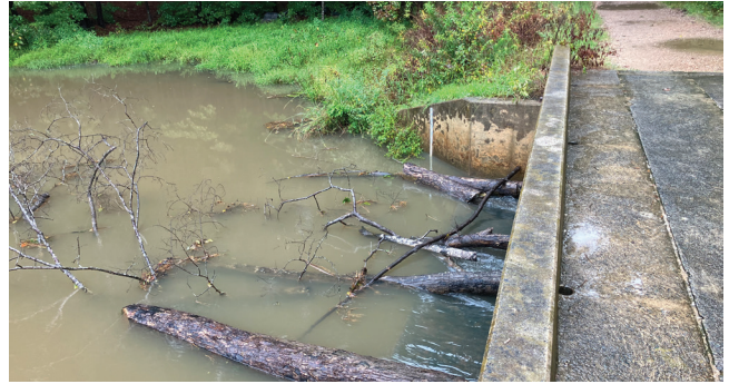
Compromised existing dam
