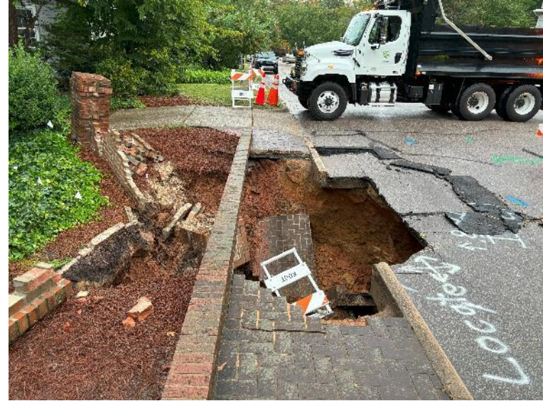
Park Drive Sinkhole
