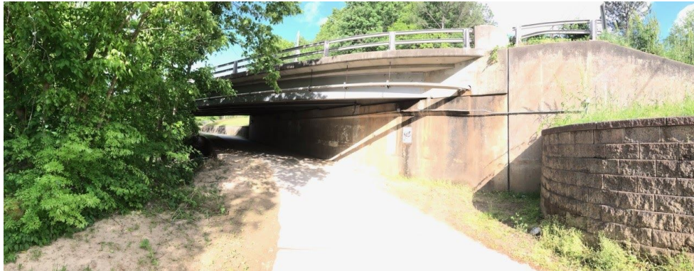
The concrete wall under the Crabtree Creek greenway off Glenwood Ave. (Located near Crabtree Mall.)
