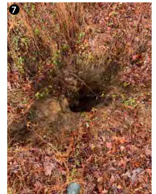
Hole in Oak Hill Drive
