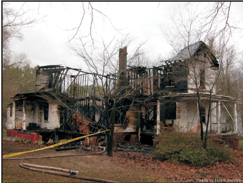
South and east elevations after fire.
