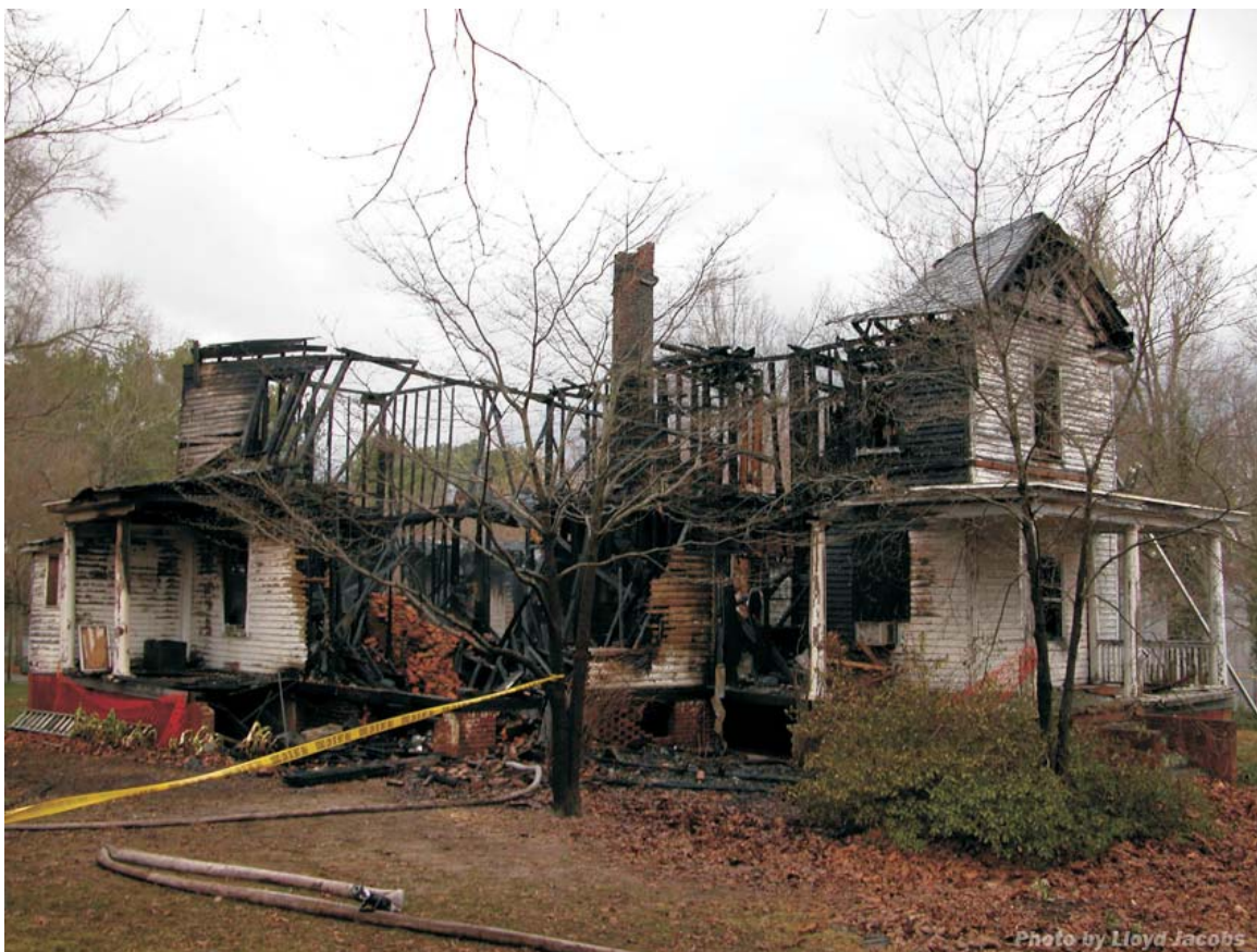
South and east elevations after fire.
