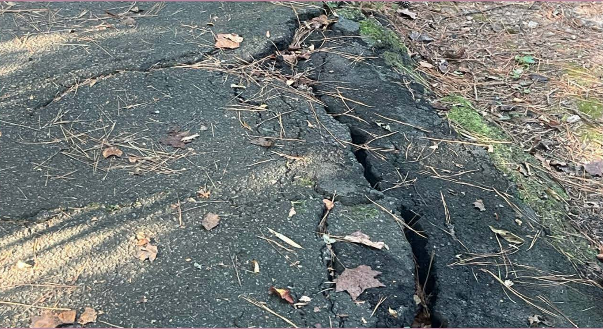
Asphalt cracking is caused by aging, root intrusion, and erosion
