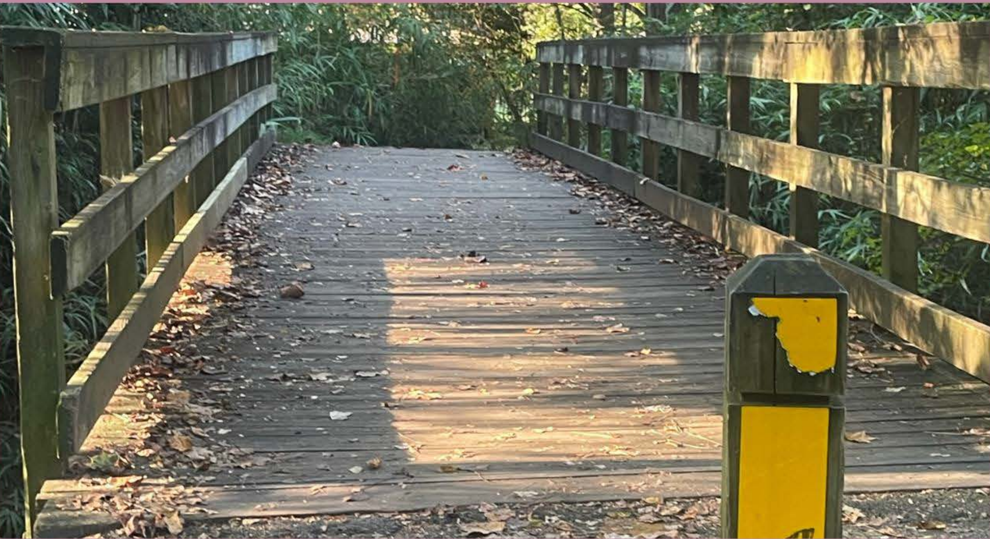
Bridges that cross Mine Creek have deteriorated
