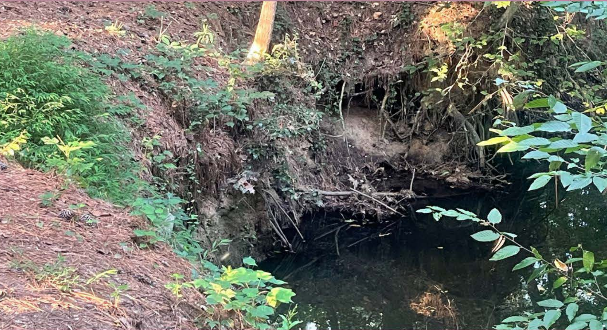
Large storm events have caused stream bank erosion, compromising the trail
