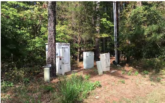
Major Utility Facilities Located Near Intersection Of Trenton Road And Reedy Creek Road Can Be Avoided.
