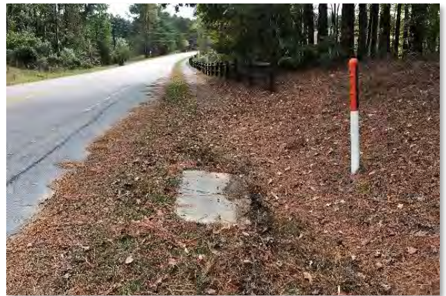
AT&T Underground Fiber Installation Near Existing Asphalt Sidewalk. Google Fiber Is Located On East Side Of Road.
