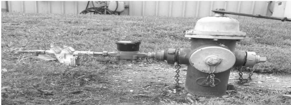
5/8" Hydrant Meters are attached directly to the fire hydrant
