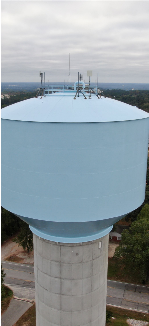
Reuse Water Tank on Sunnybrook Road
