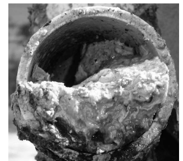
Pipe clogged with fats, oils and grease
