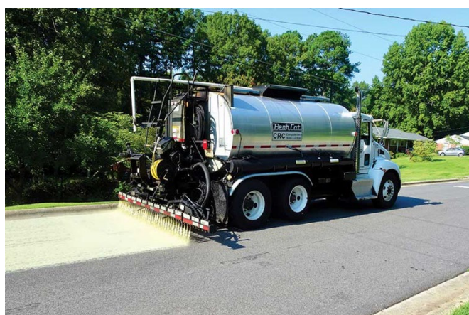
Image 16: City of Raleigh has been keeping cool! Cool roadways installation, like the one above, help the City of Raleigh reduce the impact caused by the Urban Heat Island Effect.
