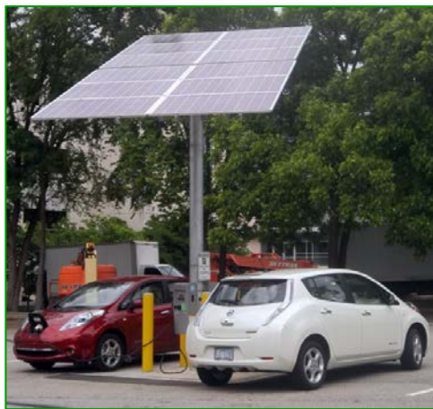
Solar EV Charging Station
