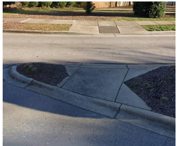
Refuge Island Ramps with Non-Compliant Width
