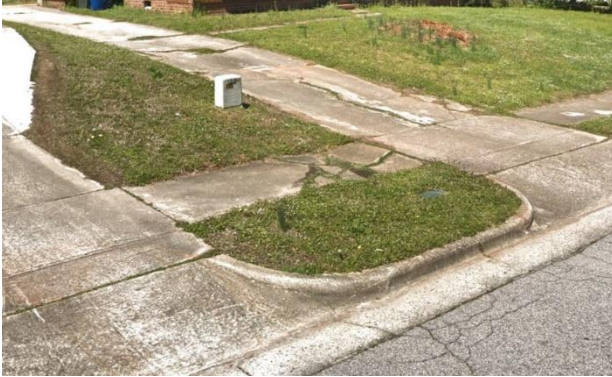
Poor Surface Condition
