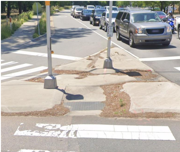
Refuge Island Ramps with Non-Compliant Run Slopes
