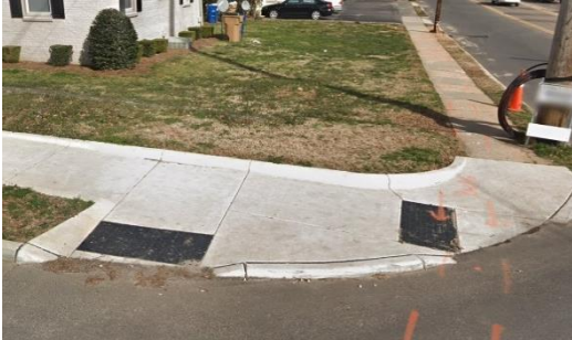
Curb Ramp Detectable Warning
