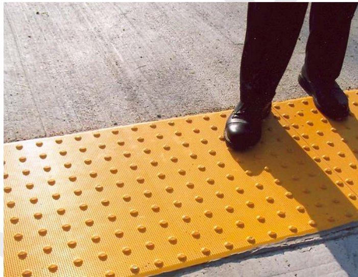
Figure 4.3 Tactile Warning Plate Example 18
